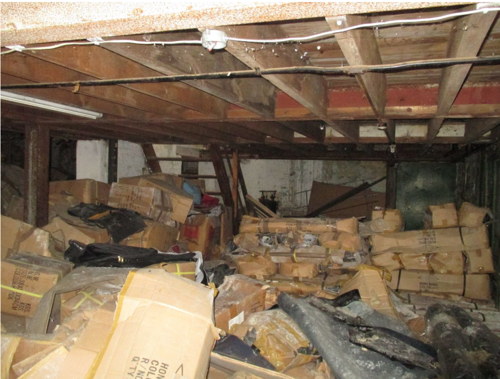
Floorspace to be demolished on northern boundary of site (Site of proposed Building C):
